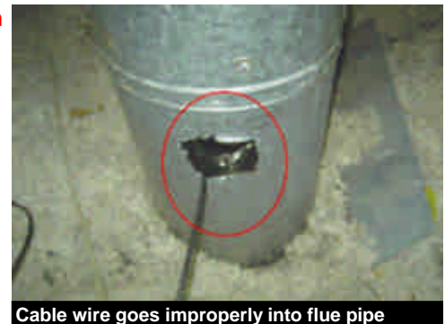
Cable wire goes improperly into flue pipe
