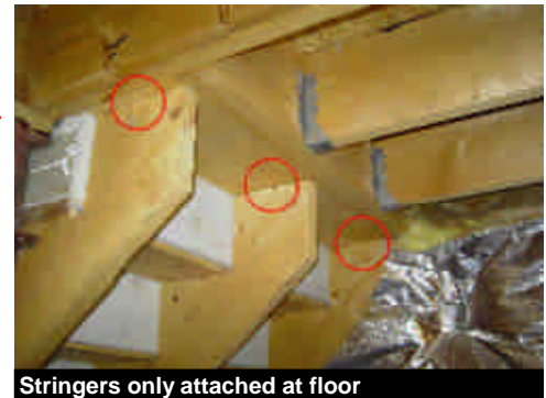
Stringers only attached at floor
