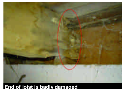
End of joist is badly damaged
