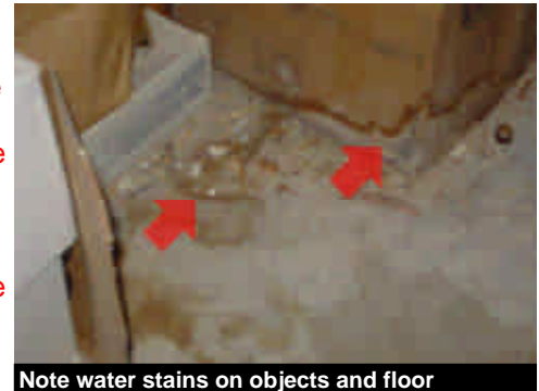
Note water stains on objects and floor
