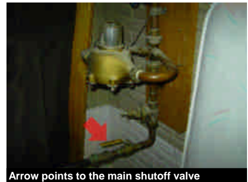
Arrow points to the main shutoff valve
