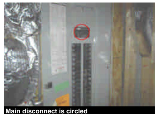
Main disconnect is circled
