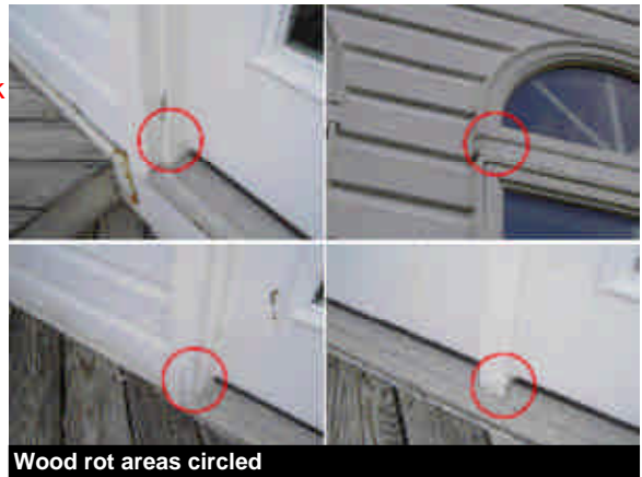
Wood rot areas circled
